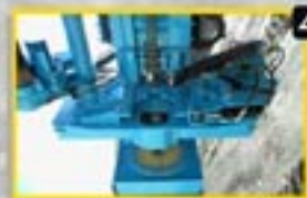
4 A complete drill table including the pick-up pot, the drill rod centralizer, a hydraulically activated pipe wrench and an automatic greaser.
